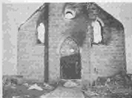
St. Mary's Church after it burned. Construction work on the church to restore it to its original beauty.
