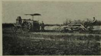
WEST BRANCH TOWNSHIP "GOOD ROAD" OUTFIT, H. H. Voth, Engineer; John H. Voth, Grader.
