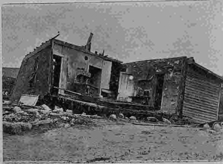
Another view of damage done by the tornadoes of June 24, 1909, discussed on the preceding page. (See also p. 155). This was the Meyers house, occupied by a Mr. and Mrs. Garrison at the time, who held the door (shown in center) shut while the tornado ripped the remainder of the house away. Miraculously, neither was injured seriously.
