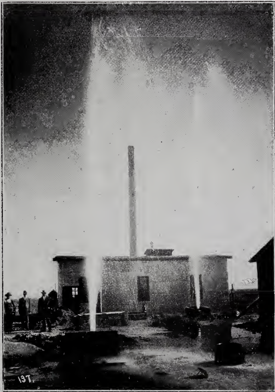
Pumping Plant Near Garden City, Kansas
