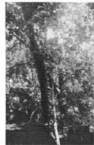
TREES ONE FOOT IN DIAMETER, Growing on top of a pier in the Ver- digris river, built in 1873, and soon to be utilized by the Kansas Railway Co. for a trolley line bridge at Altoona.
