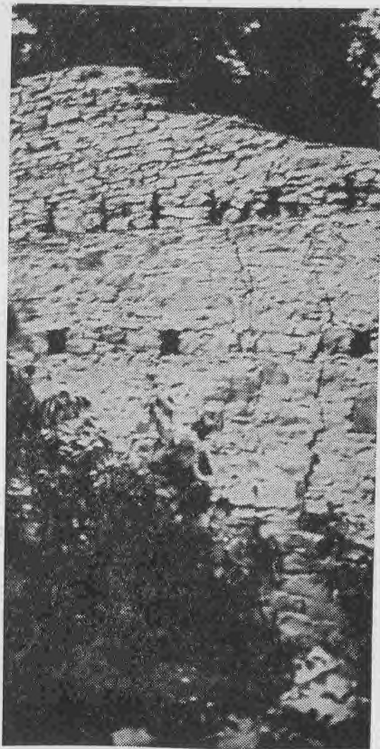
Crumbling walls of the Quindaro Hotel; the slots accepted floor timbers. Stones long since have been hauled away.
