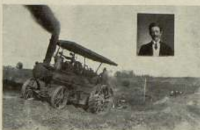
A GOOD ROAD MOVEMENT Sam Finley's Steam Tractor in action on the Cason Hill. Photograph from Sam Finley, R. F. D. 2, NEW BLOOMFIELD, MO.
