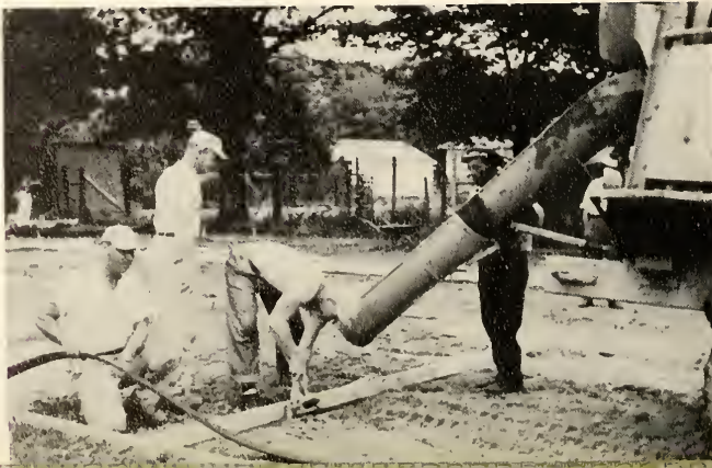
THE CONCRETE for the tennis court is poured by Otto Going, Coach Darr and Coach McGuire.
