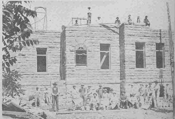
Present day court house under construction in 1899-1900. Completed June, 1900 at a cost of $30,782. Native sandstone blocks from local quarry were used in construction and this quarry is still in operation today by the Oregon-Portland Cement Company.
